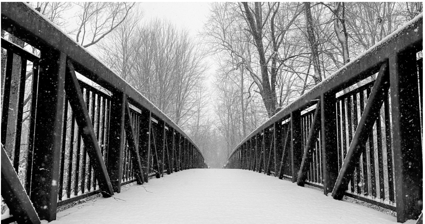
Snow on Riverside Bridge Photo credit: City of DeWitt
